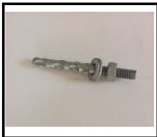
Bolts foundation indented
